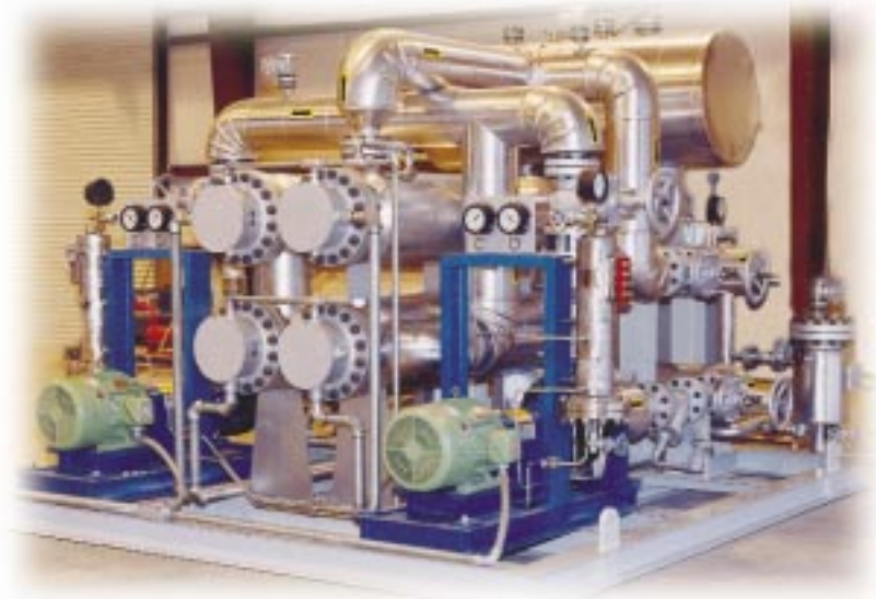
Single zone 300 kW Hot Oil System designed for installation outdoors at a petrochemical plant for heating two extruder dies. System featured 100% SCR control.
