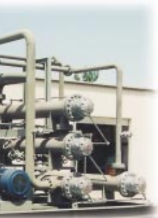
ed Hot Oil System. sed to heat extruder to
