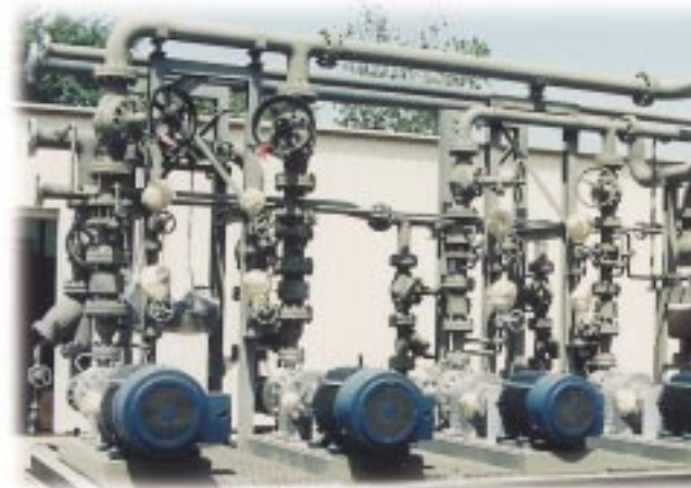
Dual zone 600 kW / 200 kW independently controlled hot oil system. Included online spare magnetic drive type pumps. System temperature 650° F. located in a petrochemical plant.
